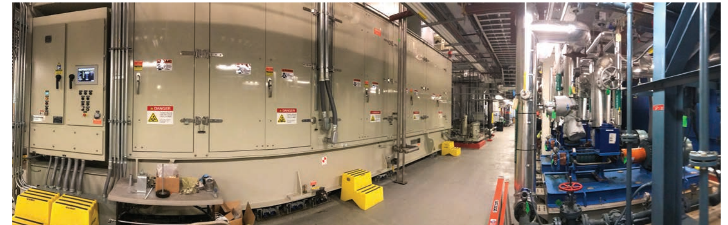
Onsite combined heat and power (CHP) plants generate electricity from natural gas and recover waste heat as usable steam and hot water. These onsite systems typically achieve a total efficiency of 70-80% and provide resiliency during power outages. We have two CHP plants on the Manhattan Main Campus, pictured here, which can produce 13.2 MW of electricity and generate enough steam for the campus' thermal needs. In addition, CHP plant at NYU Langone Hospital—Brooklyn can produce 1.6 MW of electricity and recovers heat to generate steam.
