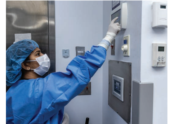
Our ventilation and HVAC setback program reduces energy use in a safe and compliant manner when select areas are occupied. This program exists in our administrative offices, research laboratories, and in our operating rooms where it saves over 3,000 MMBtu every year.
